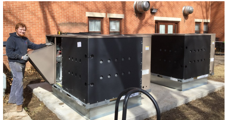
Above: Exterior Frontage of Coatsworth Apartments is directly on Galena’s Main Street; new 10-ton HVAC systems were installed, replacing circa 1968 electrical heating systems. Below: Ribbon cutting ceremony held in October 2018.
