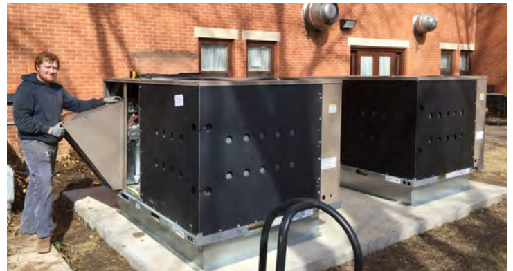
Above: Exterior Frontage of Coatsworth Apartments is directly on Galena’s Main Street; new 10-ton HVAC systems were installed, replacing circa 1968 electrical heating systems. Below: Ribbon cutting ceremony held in October 2018.
